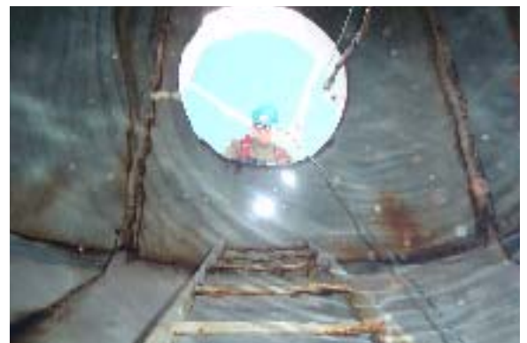
CSI's team of divers and engineers use advanced technology to inspect your reservoir and make repairs without having it drained.
