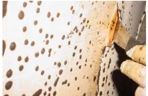
CSI can identify defective welds on wastewater liners before the system is put into service.
