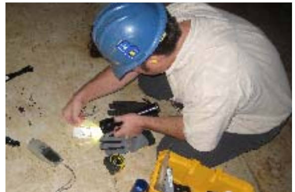
CSI determines the reason for your coating failure by conducting a detailed and thorough on-site investigation and methodical assessment.
