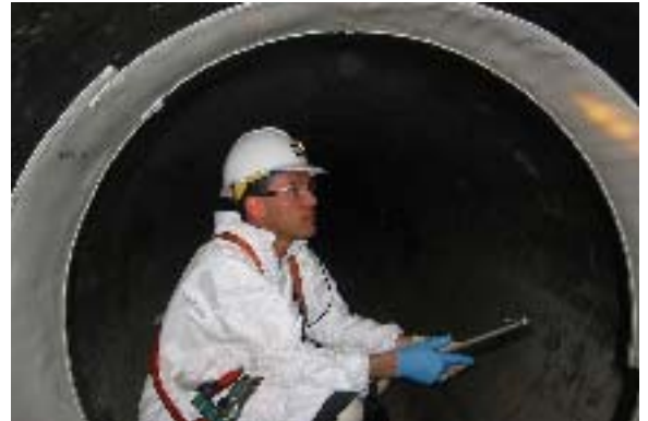
Skilled inspectors scrutinize PVC liner welds and seams to determine proper installation.
